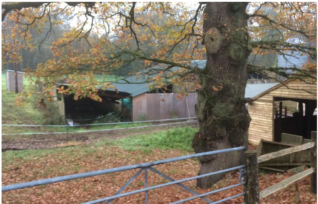
Figure 5: Timber shed and lean-to (Barn B) in relationship to veteran oak tree. (150 -300years old). It also shows the recent substantial infilling of the walls in progress and new metal profile roofing. Unauthorized 'works' despite a Planning Contravention Notice (PCN) 2020.
